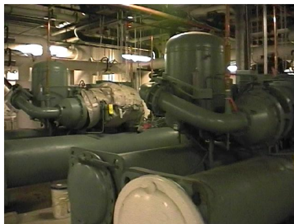
Figure 3: Two 15-Ton Chillers
